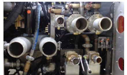
Multiple plumbing possibilities
